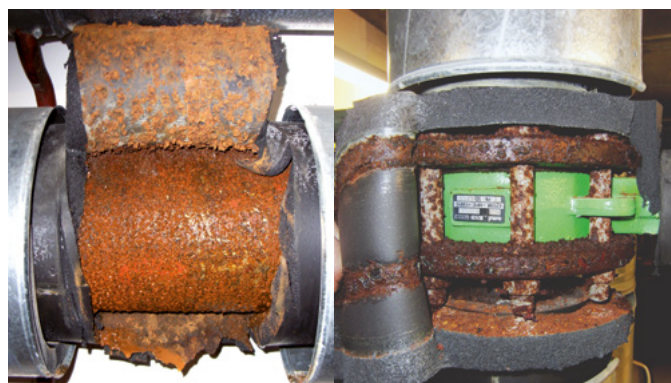
corroded steel pipes
