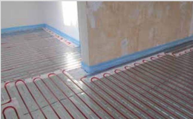
Completed heating system TS
