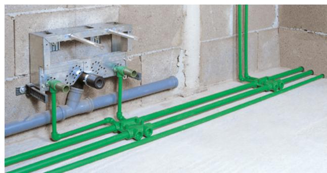
Floor distribution with distribution blocks
