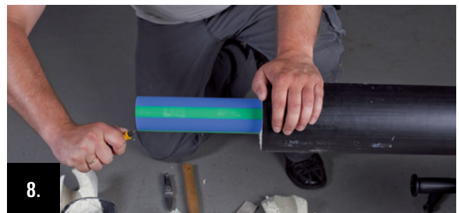
8. Clean the skinned medium pipe and deburr the pipe ends inside and outside.
