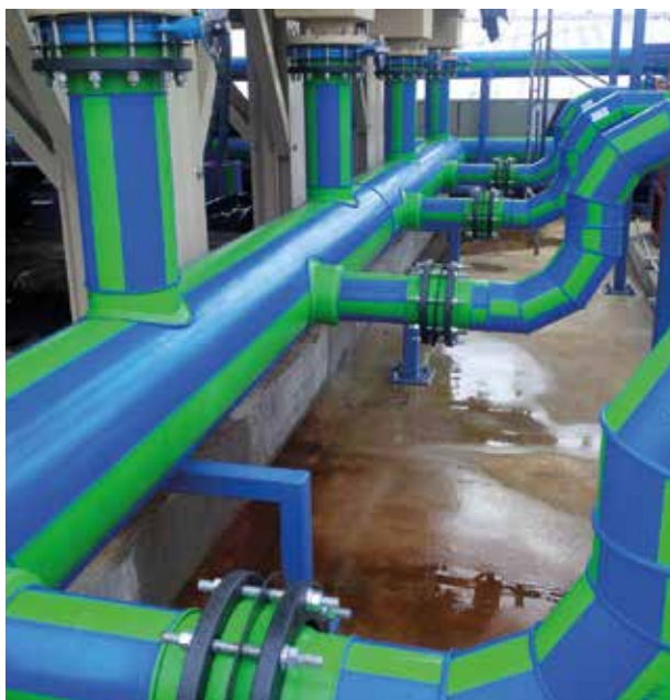
Supply process cooling
