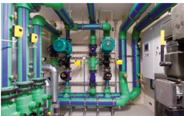
Heating manifold under-soil heating
