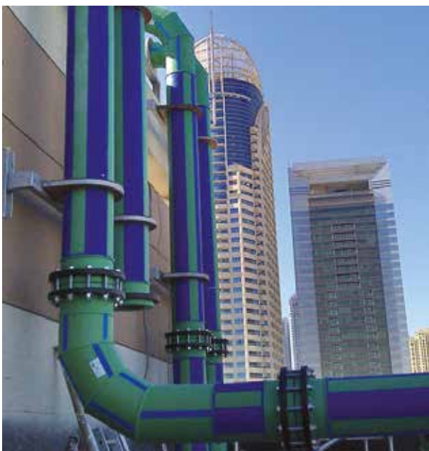
Supply process cooling
