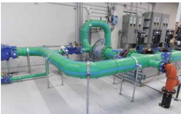
Drinking water pressure increase
