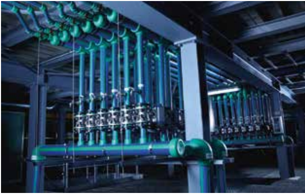
Mixing plant for industrial fluids
