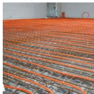
Industrial floor heating
